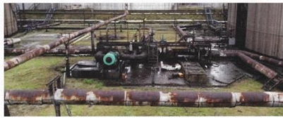
Figure 1. Decontamination methodologies should be carefully considered on disused oil storage sites and distribution terminals.
