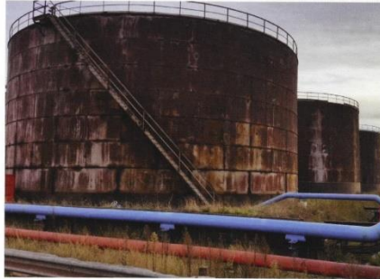
Figure 3. Redundant tanks ready for decommissioning.
